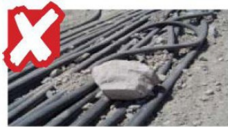
Figure 7: Example of rocks gathering on cables
