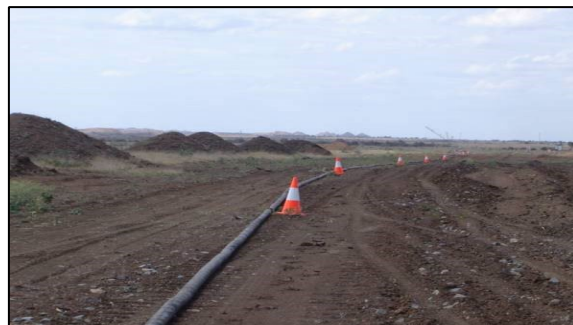
Figure 19: Good standard for cable route.
