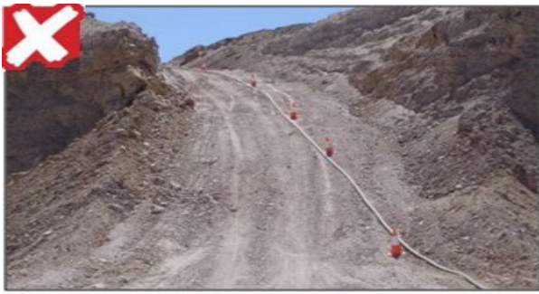
Figure 18: Poor standard of cable route, not wide enough.
